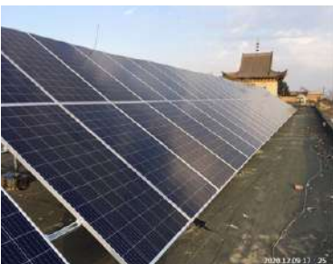
Solar power for a primary school in China, 2021
